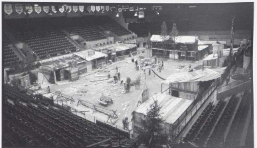
Work in Progress: Construction during Ball Week continues before, after and during class.
