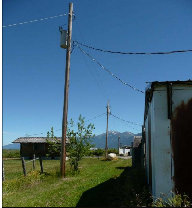
Figure 6. View to the North of the Power-line Transformers
