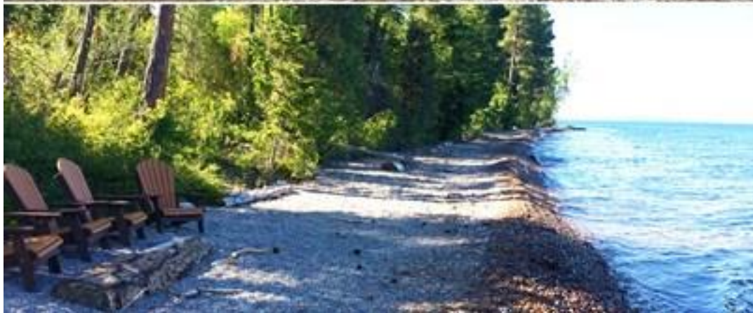
These images show the progression from the original shoreline (top image, with original waterline shaded in blue), through snowy construction in the spring (middle image), to the newly restored gravel beach shoreline (bottom image).
