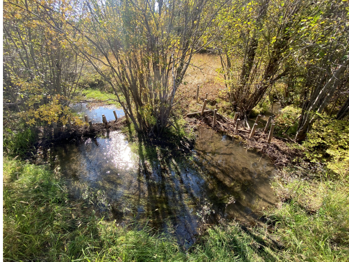
Figure 1: Beaver dam analogs constructed on Fish Creek, Montana in Fall 2019 using wooden posts and interwoven conifers. Photo credit: Ben Colman.
