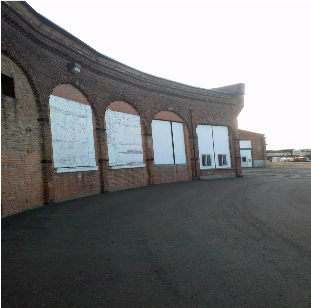
Another view of the roundhouse in Glendive shows the original brickwork in the arches, filled in over time with new brick.
