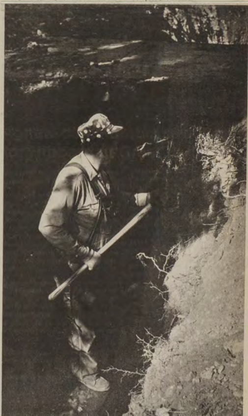
AN EMPLOYEE of 4-G and Lembke Plumbing and Heating, works on an extension of the University of Montana water line system on East Beckwith Avenue. J. "Ted" Parker, director of the UM Physical Plant, said the Montana Power Company water main will probably be completed and the street reopened next week. (Montana Kaimin photo by Randy Rasmussen.)
