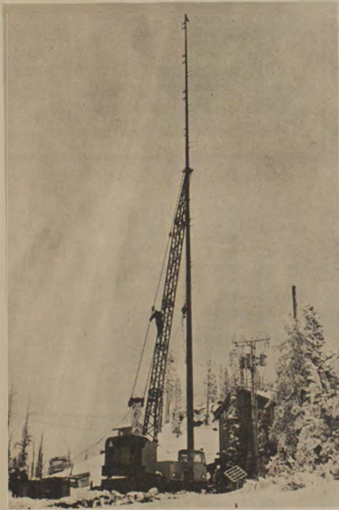
NOT RAIN NOR SNOW nor dark of night . . . or so goes the saying. The KUFM radio antenna seen here will soon be completed and ready for use. The antenna is on top of Big Sky Mountain, 11 miles north of Missoula. (Photo by Joe Stark)
