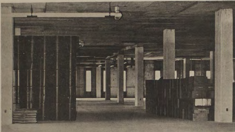
IF YOU HAVE been having problems finding books on the lower two levels of the new library, you would be in for even greater troubles on the top two floors. Awaiting completion, these two levels are currently being used to store such items as these civil defense air raid shelter supplies. (Montana Kaimin photo by Gary MacFadden)
