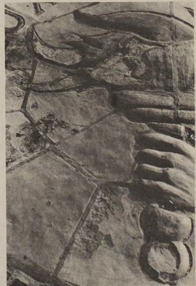
CRACKING AND CHIPPING of the clay design in the center of the oval is a result of not firing the clay at a high enough temperature, say artists Arne Autio and John McCoy. Water freezing in the design continues its damage. No funds are available for the repair of the $2,000-plus design which took two months to build. (Montana Kaimin photo by Tom Levno)
