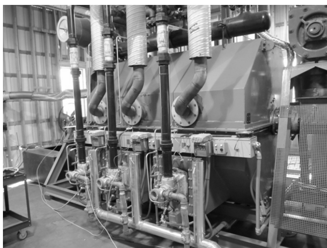
Figure 1. The Tucker Engineering Associates (TEA) gasifier used in this study. Photo: RMRS.
